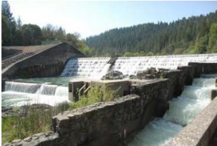
VICINITY MAP OF VAN ARSDALE FISHERIES STATION/RESERVOIR and PHOTO OF CAPE HORN DAM
